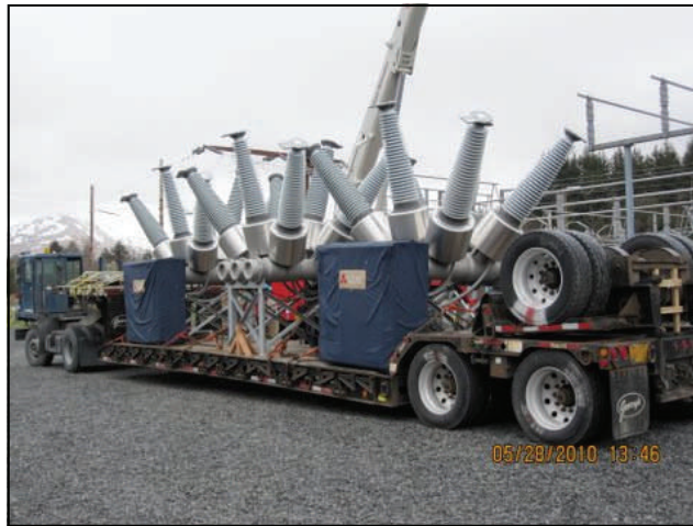
New "oil free" SF6 138 KV breakers are transported by semi-trailer to Airport Substation
